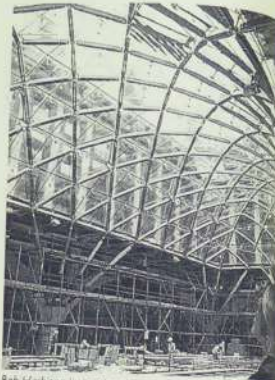
Bob Harbison inspecting the eccentric new Parliamentary Building by Michael Hopkins, now nearing completion.
